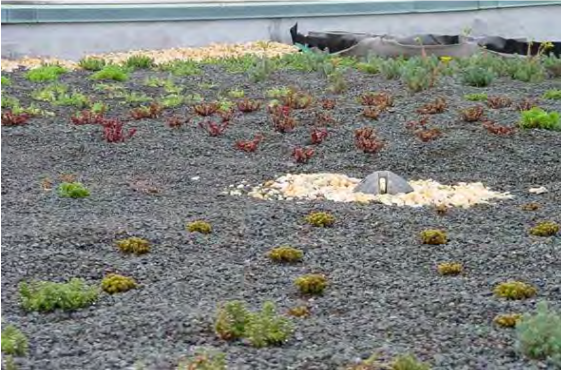
Figure 4-13. White gravel indicates a no plant zone for a green roof, Raleigh, North Carolina. Source City of Raleigh
