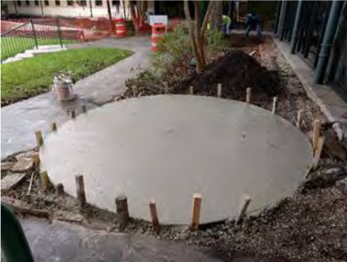
Figure B-9-4. Construction of a concrete foundation for cistern at San Antonio River Authority Main Office, San Antonio, Texas.
