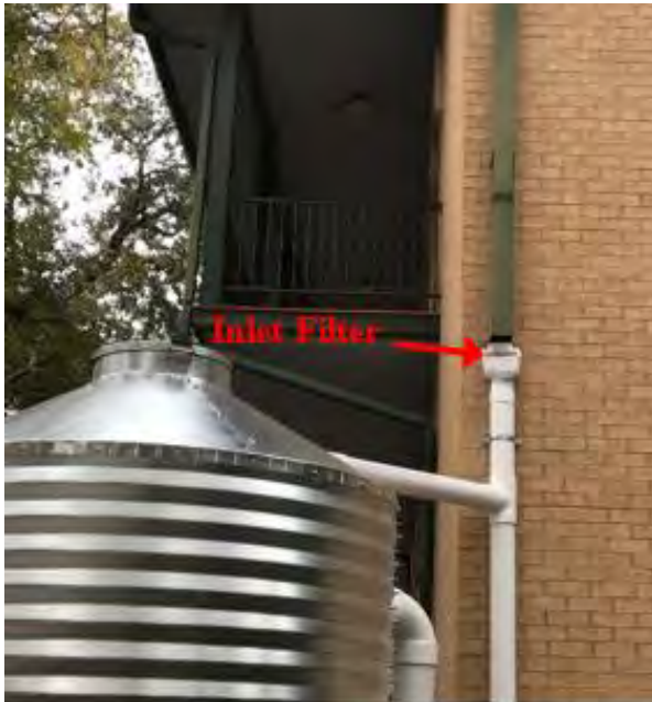
Figure B-9-10. Inlet filter at the gutter at San Antonio River Authority Main Office, San Antonio, Texas.
