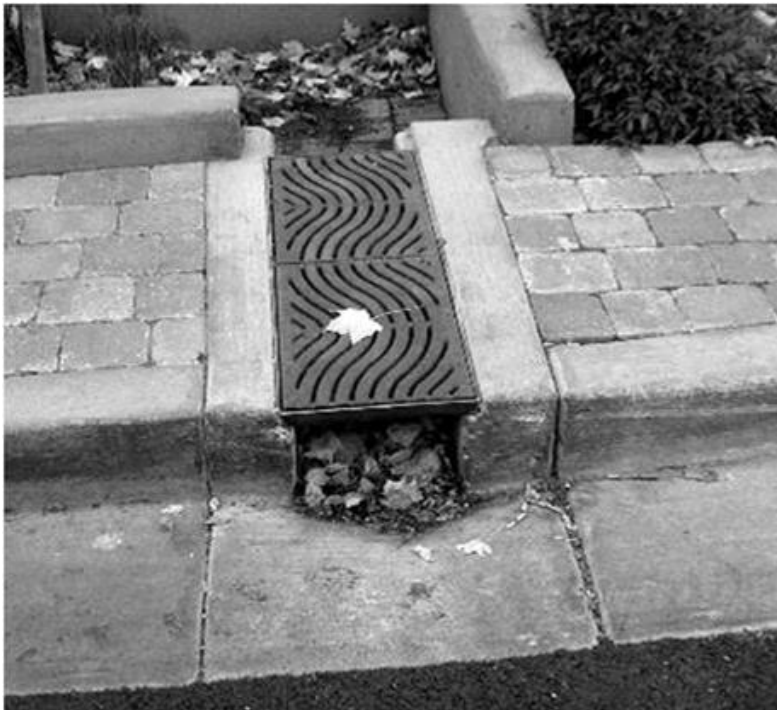
Figure 4-7. Inlet sump to remove gross solids. Source: Portland Bureau of Environmental Services
