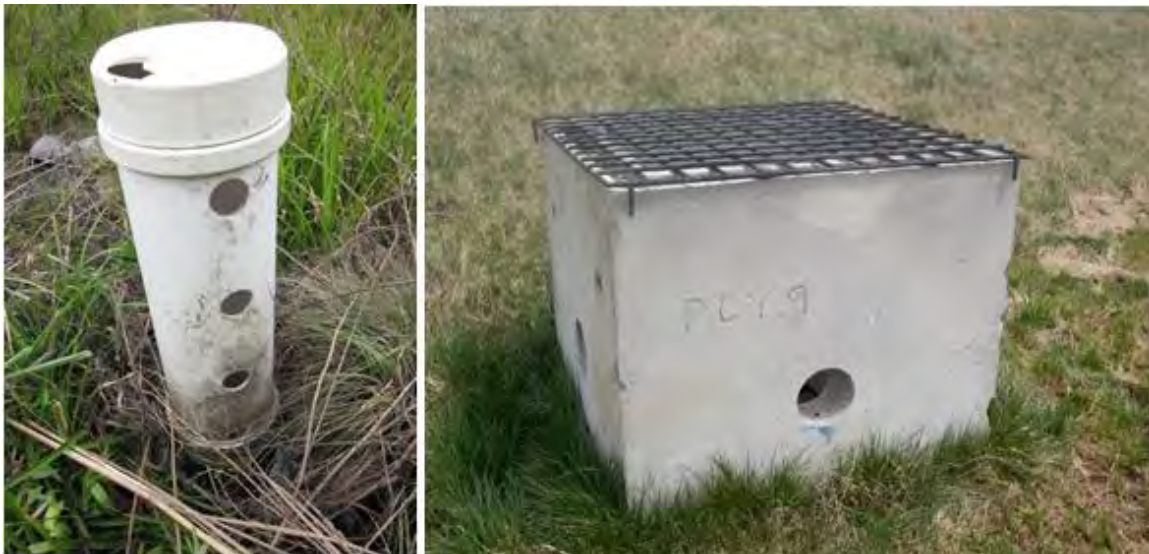
Figure B-1-11. Bioretention outlet structures designed for peak flow mitigation in Camp Pendleton, California (left) where a graduated riser pipe regulates drawdown of the detention volume; and Southwest Middle School, Gastonia, North Carolina (right) where orifices allow controlled dewatering of the detention volume and water quality treatment volume is retained below the orifice elevation. Source: Tetra Tech
