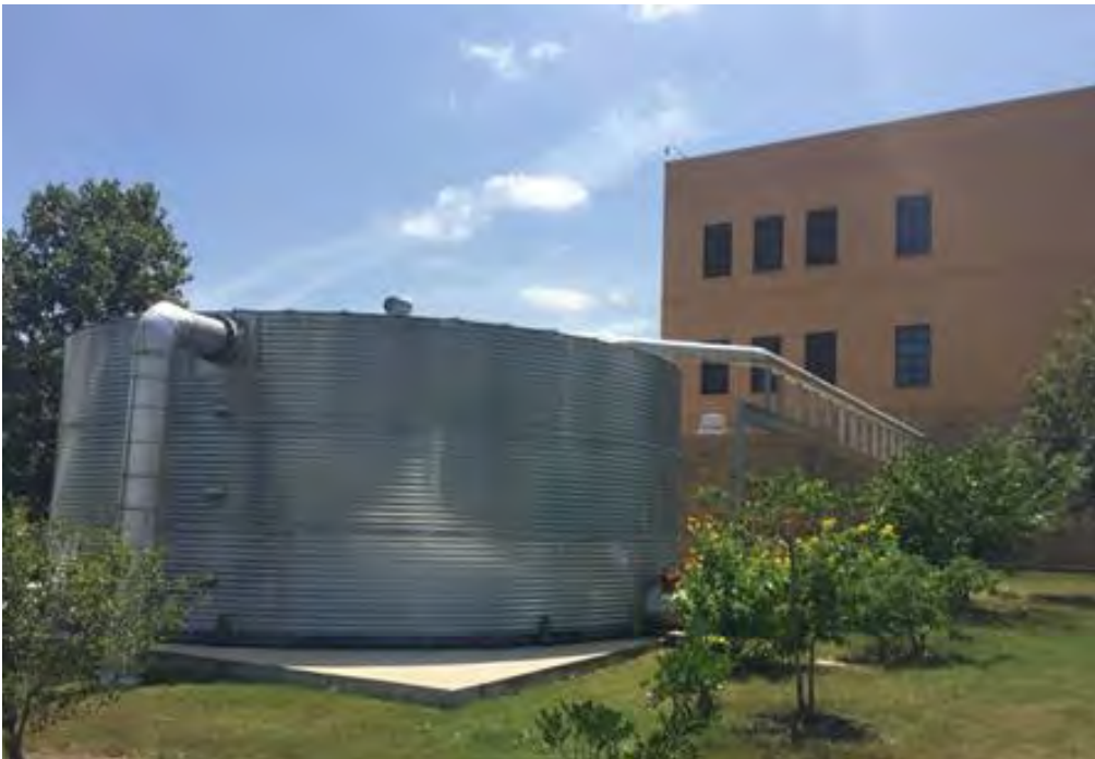
Figure B-9-6. Inlet in the top of the cistern at Texas A&M University at San Antonio, San Antonio, Texas.
