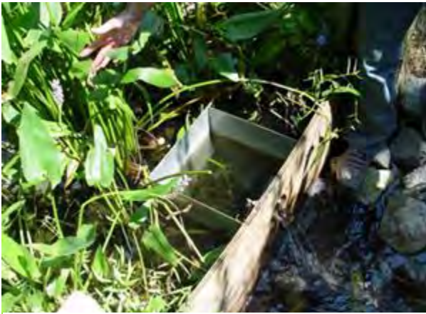
Figure 4-12. Outlet with a trash rack. Source North Carolina State University Department of Biological and Agricultural Engineering
