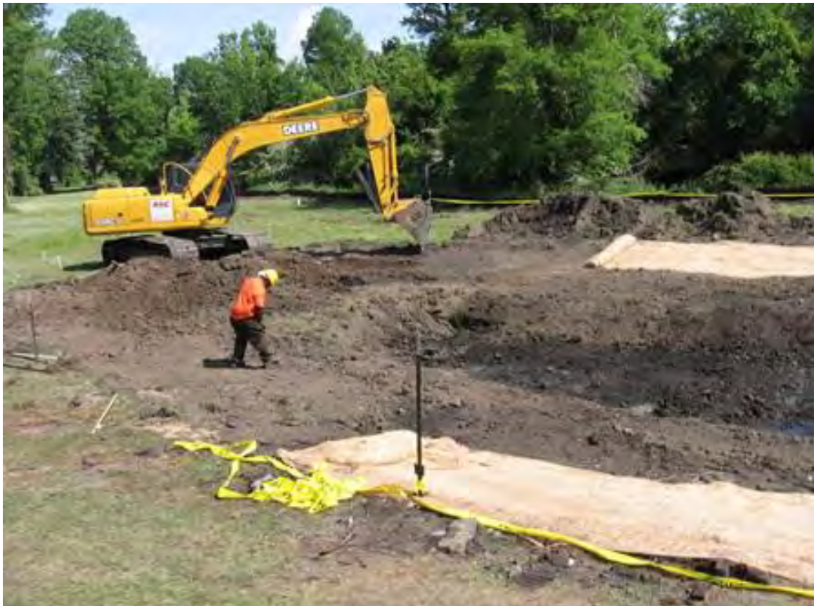
Figure 4-4. Heavy equipment being operated outside the excavated area to prevent compaction. Source: Tetra Tech
