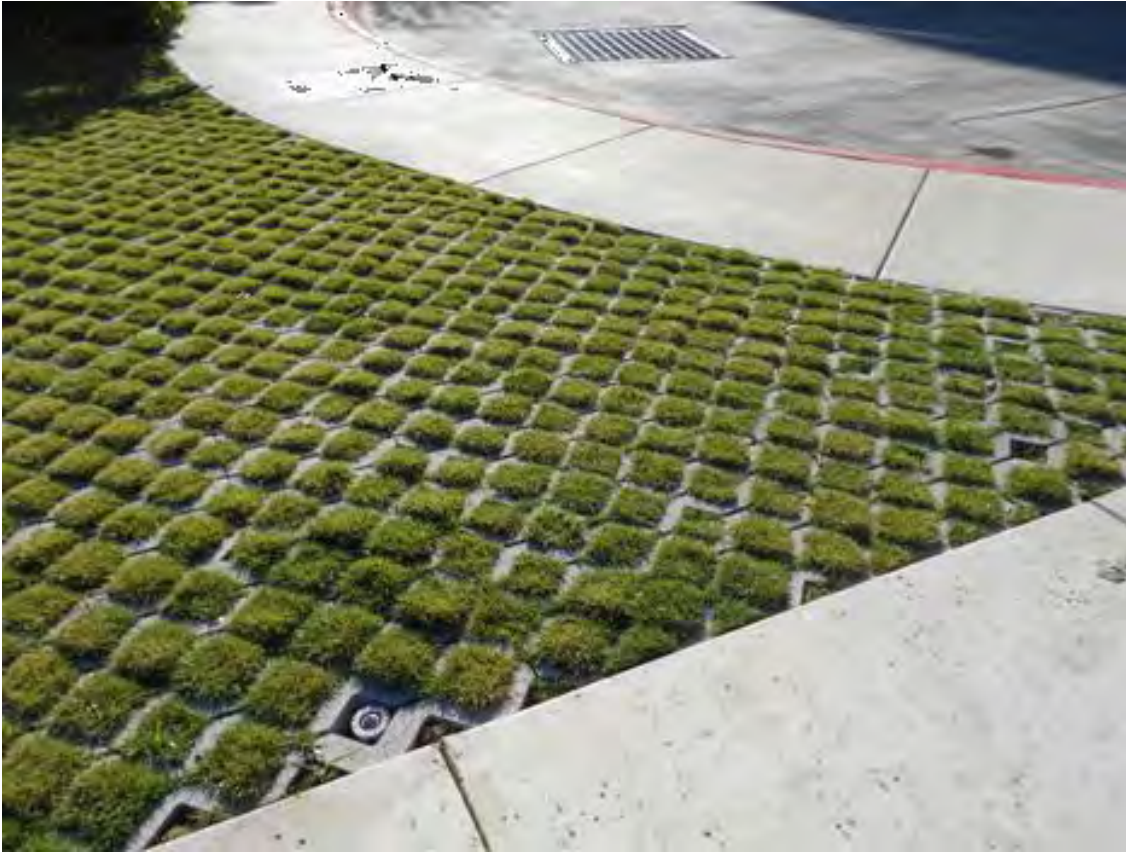
Figure B-3-8. Example of Concrete Grid Pavers (CGP) planted with turf grass that serves as an emergency vehicle access and landscape feature at the River House, San Antonio, Texas.
