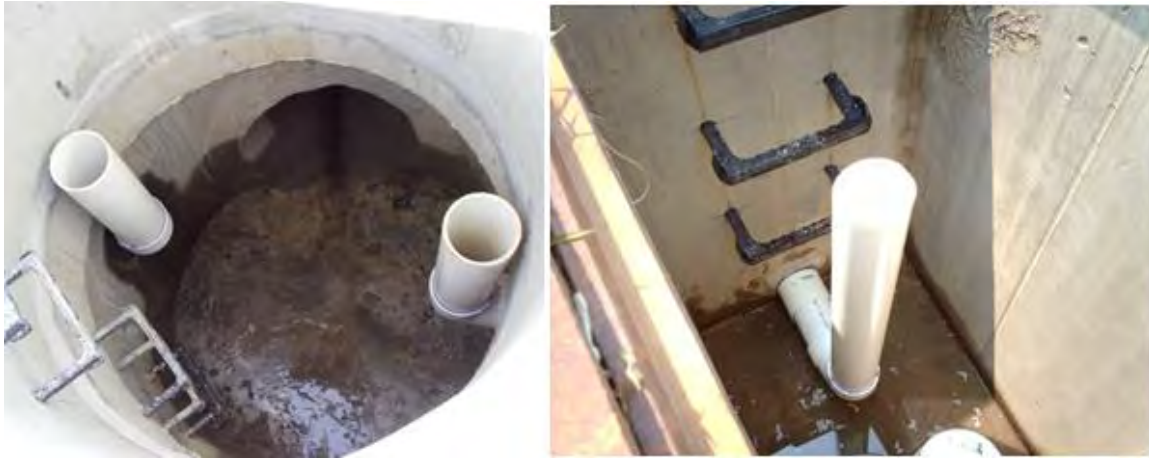
Figure B-1-4. Upturned underdrains inside bioretention outlet structures create IWS in soil media to improve infiltration, water quality, and plant health, North Carolina. Source: Tetra Tech
