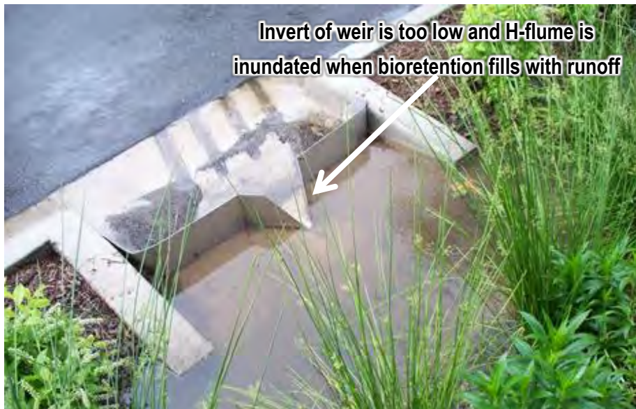
Figure 4-20. Poorly installed H-flume at the inlet to a bioretention area in which the invert of the weir is too low and tailwater from the bioretention will interfere with measurement. Source: Tetra Tech
