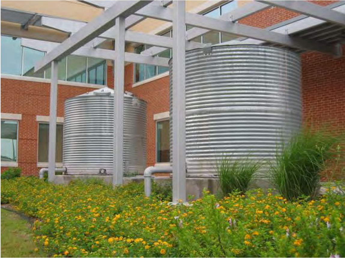
Cisterns at Cliff Morton Development and Business Services Center, San Antonio, Texas. Source: Bender Wells Clark Design
