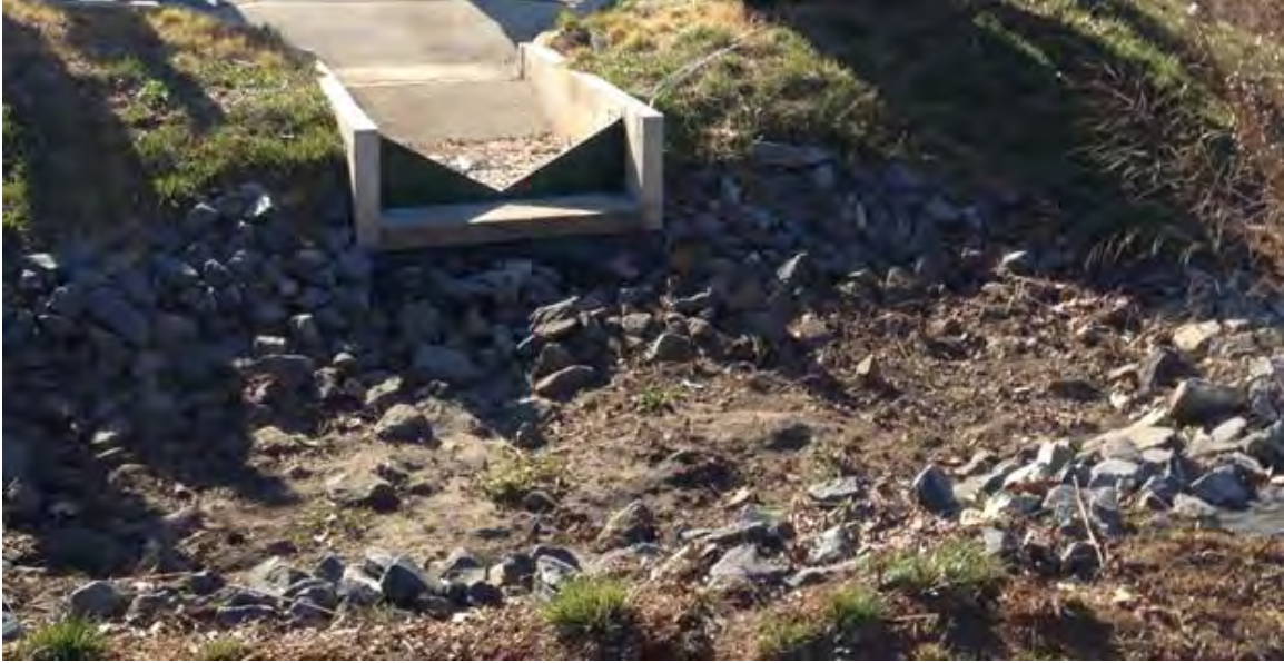
Figure 4-16. Inlet curb cut with a v-notch weir. Source: Tetra Tech
