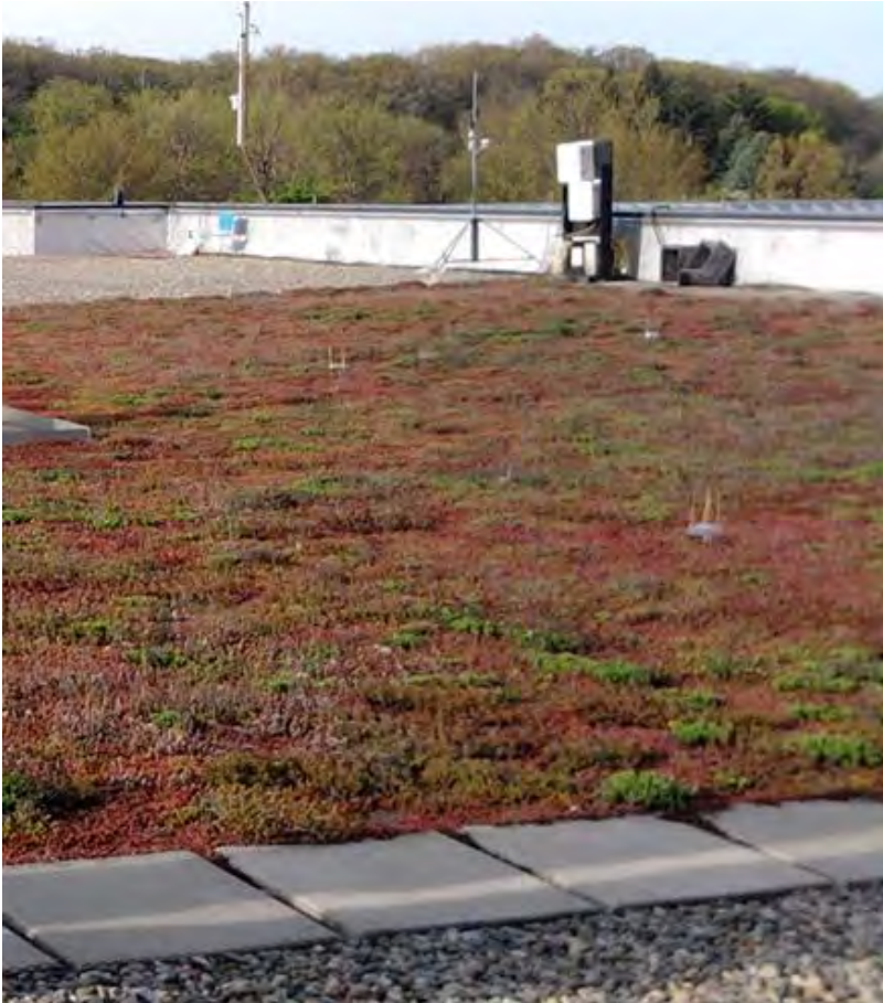
Figure B-5-1. Example of an extensive green roof, East Lansing, Michigan. Source: Tetra Tech
