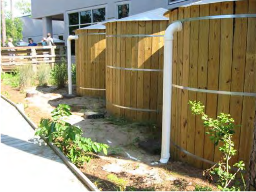
Figure 3-22. Wood wrapped cisterns, Pine Knoll Shores, North Carolina. Source: Tetra Tech
