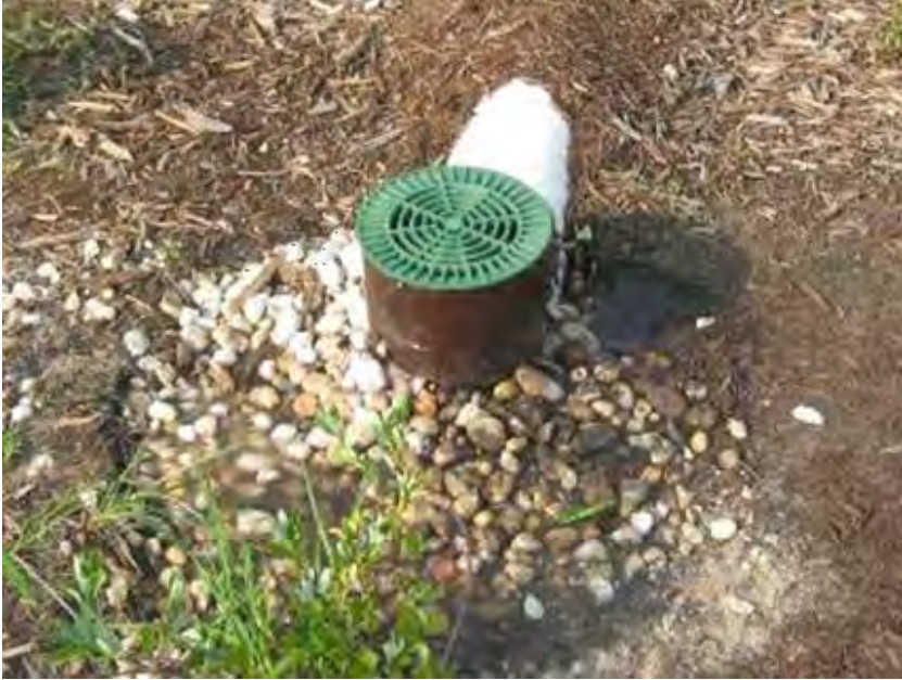
Figure B-13-9. Upturned roof downspout energy dissipater, Chocowinity, North Carolina. Source: Tetra Tech
