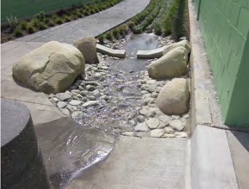
Figure B-1-6. Inlet and pretreatment provided by mortared cobble forebay and energy dissipater, Los Angeles, California. Source: Tetra Tech
