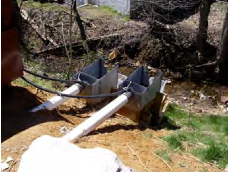
Figure 4-18. Underdrains from permeable pavement equipped with 30° V-notch weir boxes and samplers for flow and water quality monitoring. Source: Tetra Tech
