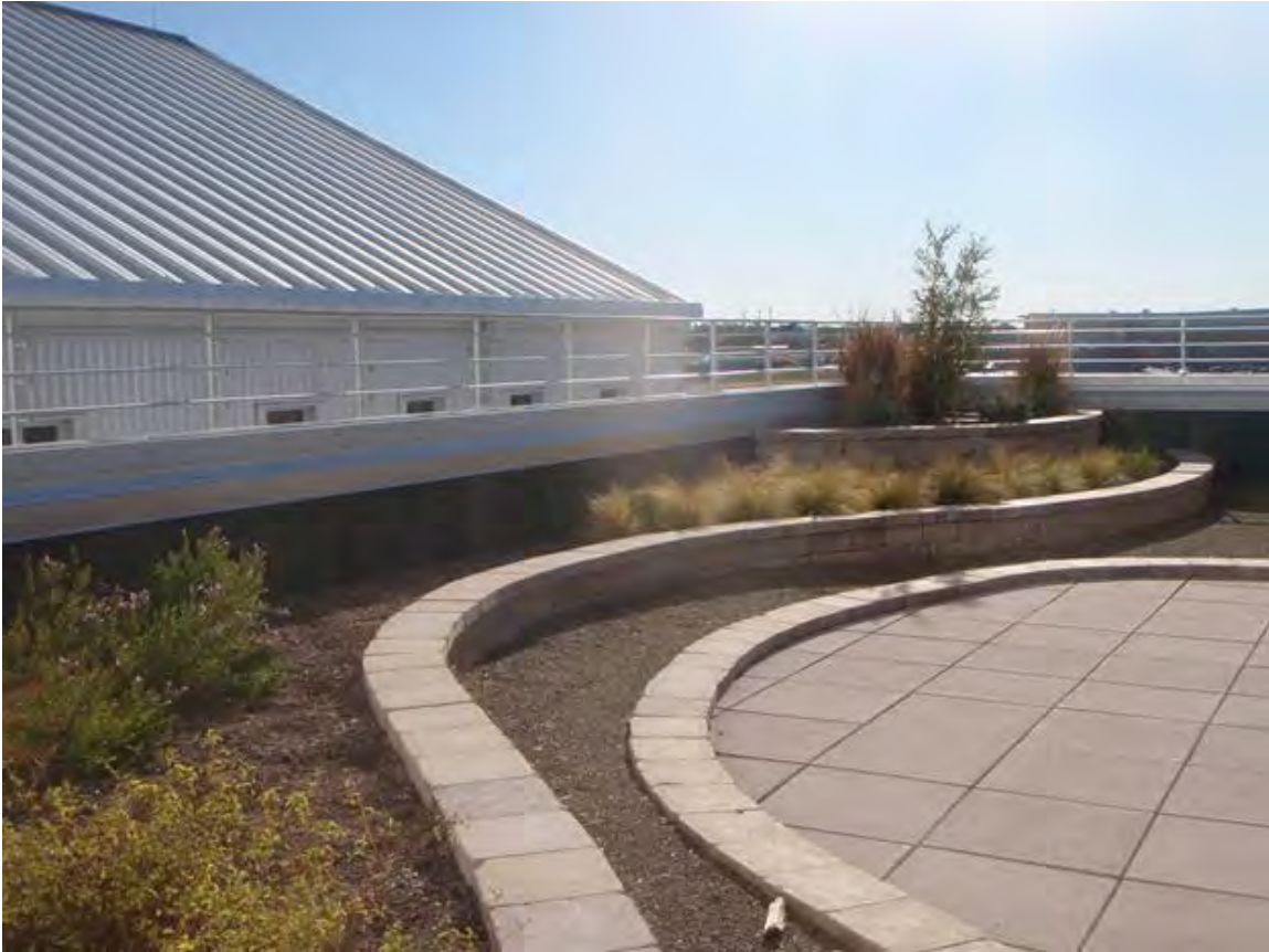
Figure B-5-5. Green roof that provides educational and recreational opportunities at James Madison High School Agriscience Building, San Antonio, Texas. Source: Bender Wells Clark Design
