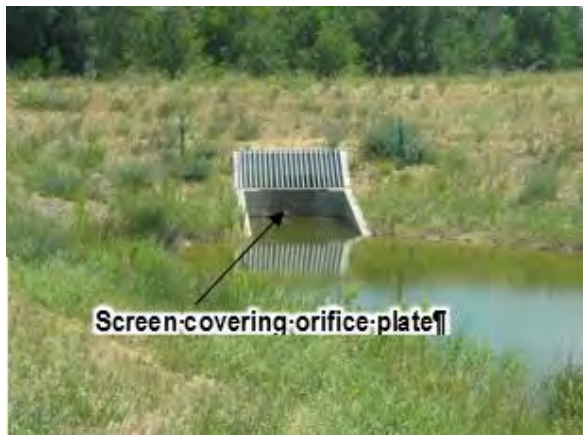
Figure B-8-7. Sloped trash rack with parallel wing walls. Source: Urban Drainage Flood Control District
