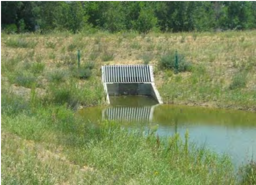
Figure 4-14. Sloped trash rack with parallel wing walls. Source: Urban Drainage Flood Control District
