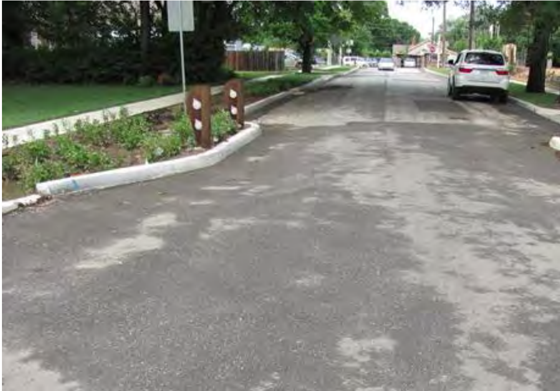
Figure 1-15. Bioretention incorporated into a pop-out, Kansas City, Missouri. Source: Tetra Tech
