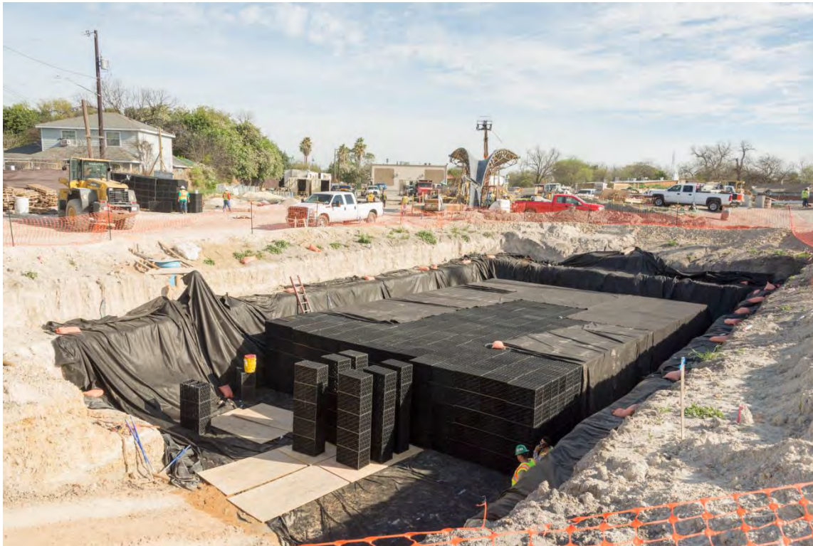
Figure 3-24. Large below ground cistern under construction, Confluence Park, San Antonio, Texas. Source: San Antonio River Foundation
