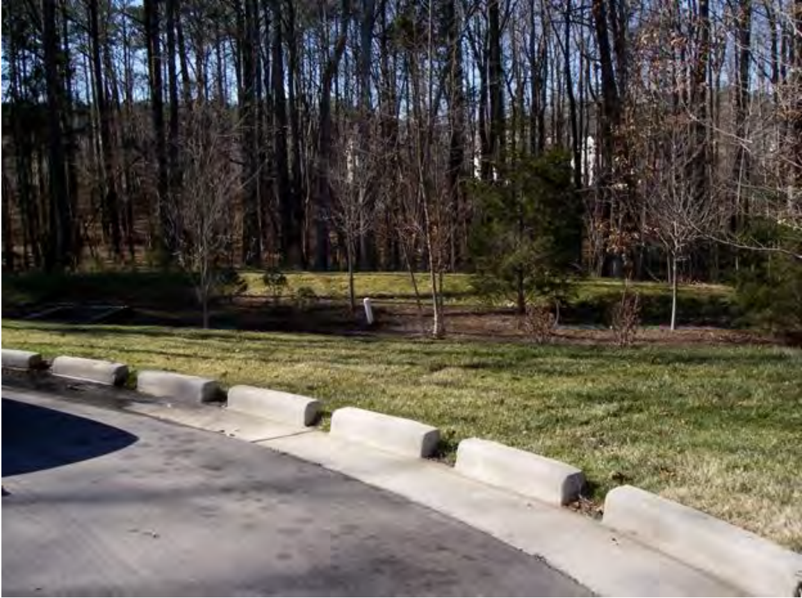
Figure 3-31. Vegetated filter strip that pretreats roadway runoff, Apex, North Carolina. Source: Tetra Tech
