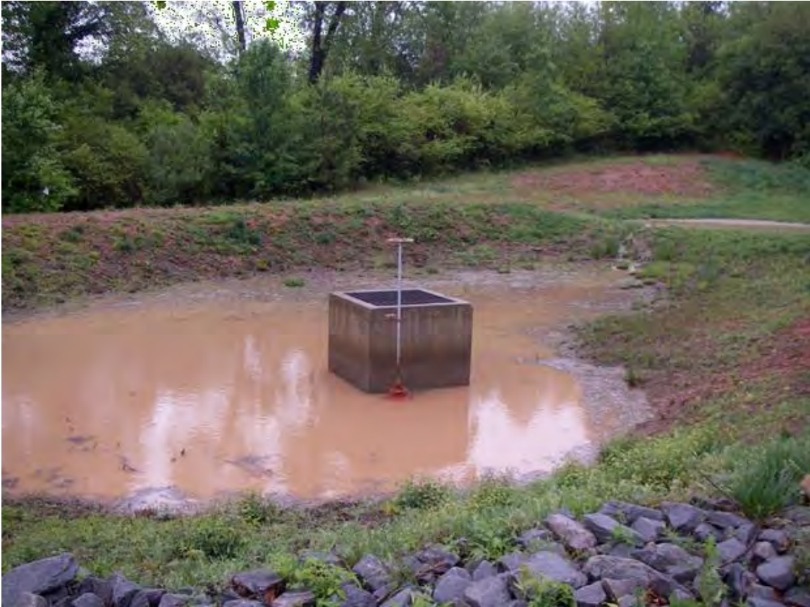
Figure B-7-10. Maintenance dewatering intake design that could be used in a stormwater wetland, Raleigh, North Carolina. Source: Tetra Tech
