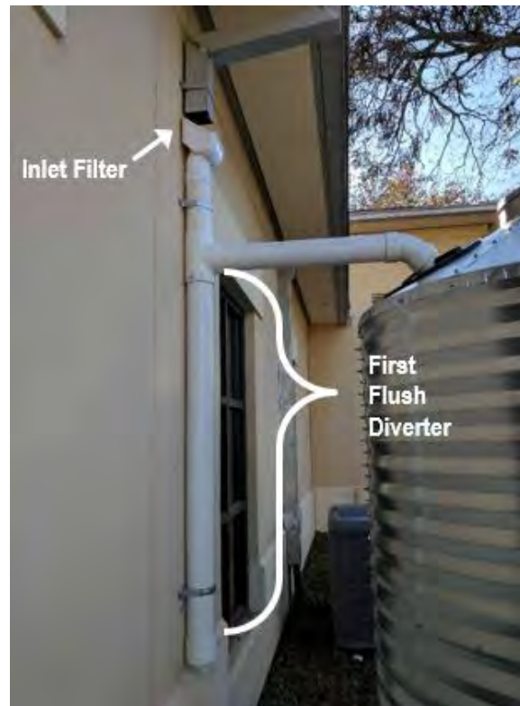
Figure B-9-15. First-flush diverter configuration at the downspout at San Antonio River Authority Main Office, San Antonio, Texas.
