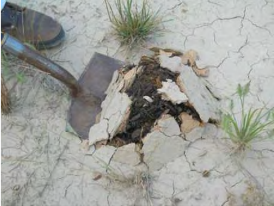
Figure 4-6. Bioretention area clogged with sediment. Source North Carolina State University Department of Biological and Agricultural Engineering
