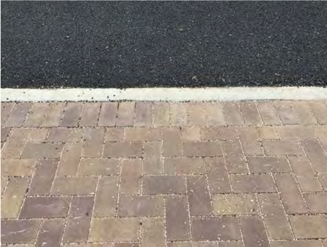
Figure B-3-14. A 1-foot concrete transition strip is used as an edge restraint between PCIP and impermeable asphalt, Floresville, Texas.
