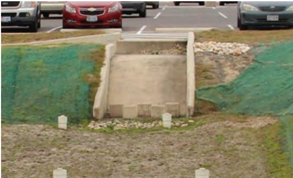
Figure B-13-8. Concrete energy dissipater, University of Texas at San Antonio, San Antonio, Texas. Source: Tetra Tech
