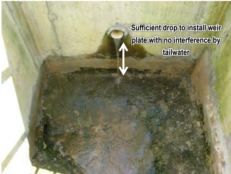
Figure 4-19. Example of a bioretention underdrain outlet with sufficient drop to install a flow monitoring weir without encountering tailwater. Source: Tetra Tech
