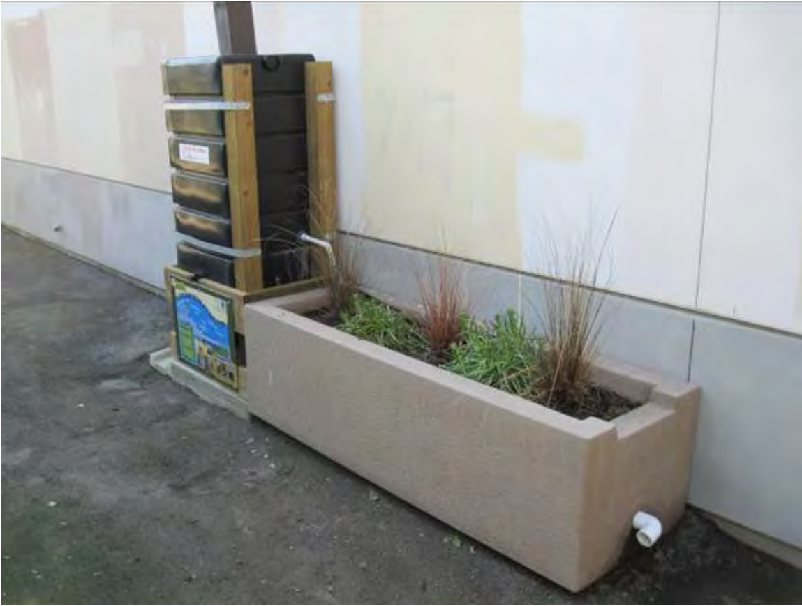
Figure B-9-16. Cistern outlet into a planter box in San Diego, California. Source: Tetra Tech
