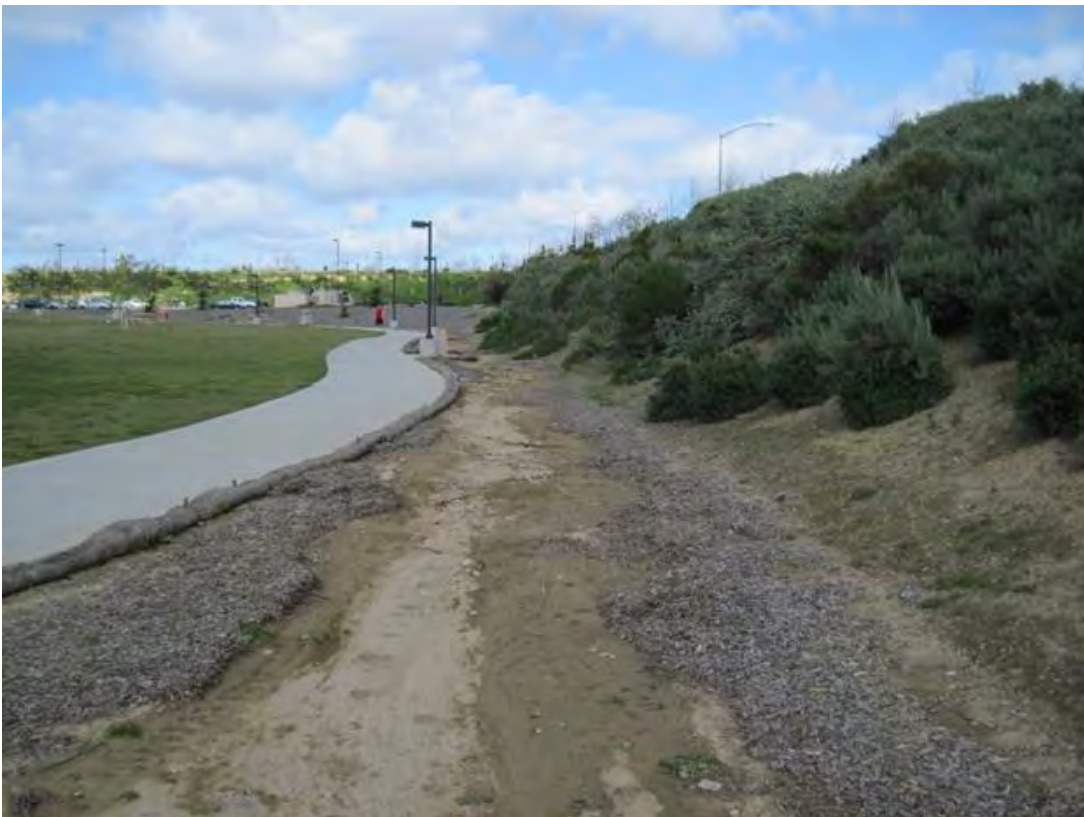
Figure 4-8. Erosion caused by excessive flows in a bioswale. Source: Tetra Tech
