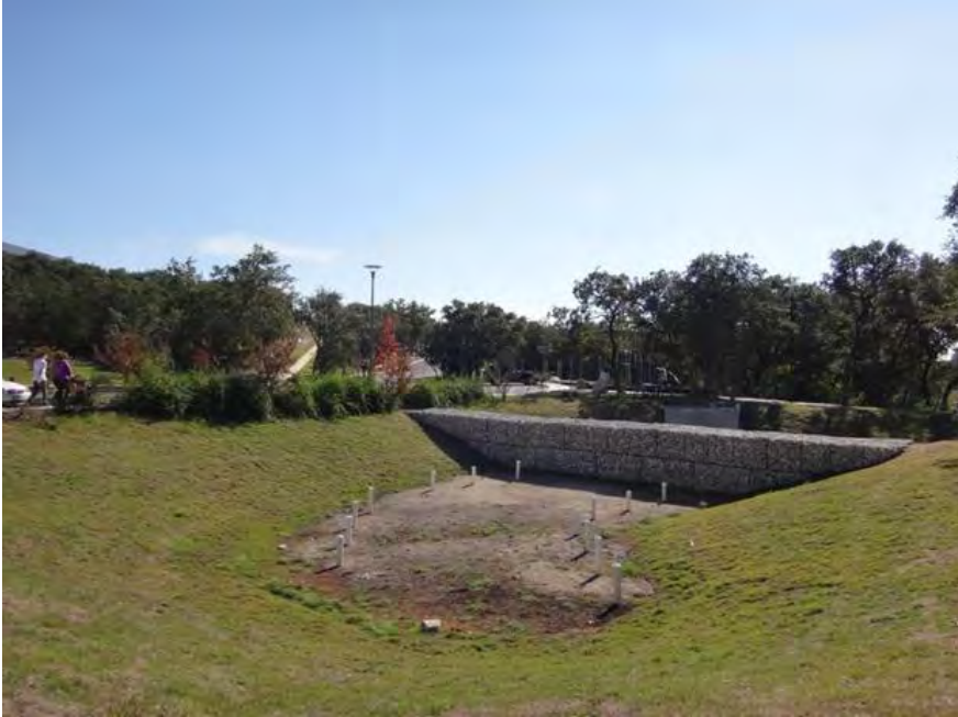
Figure B-6-1. Surface sand filter at Parman Library, San Antonio, Texas. Source: Bender Wells Clark Design
