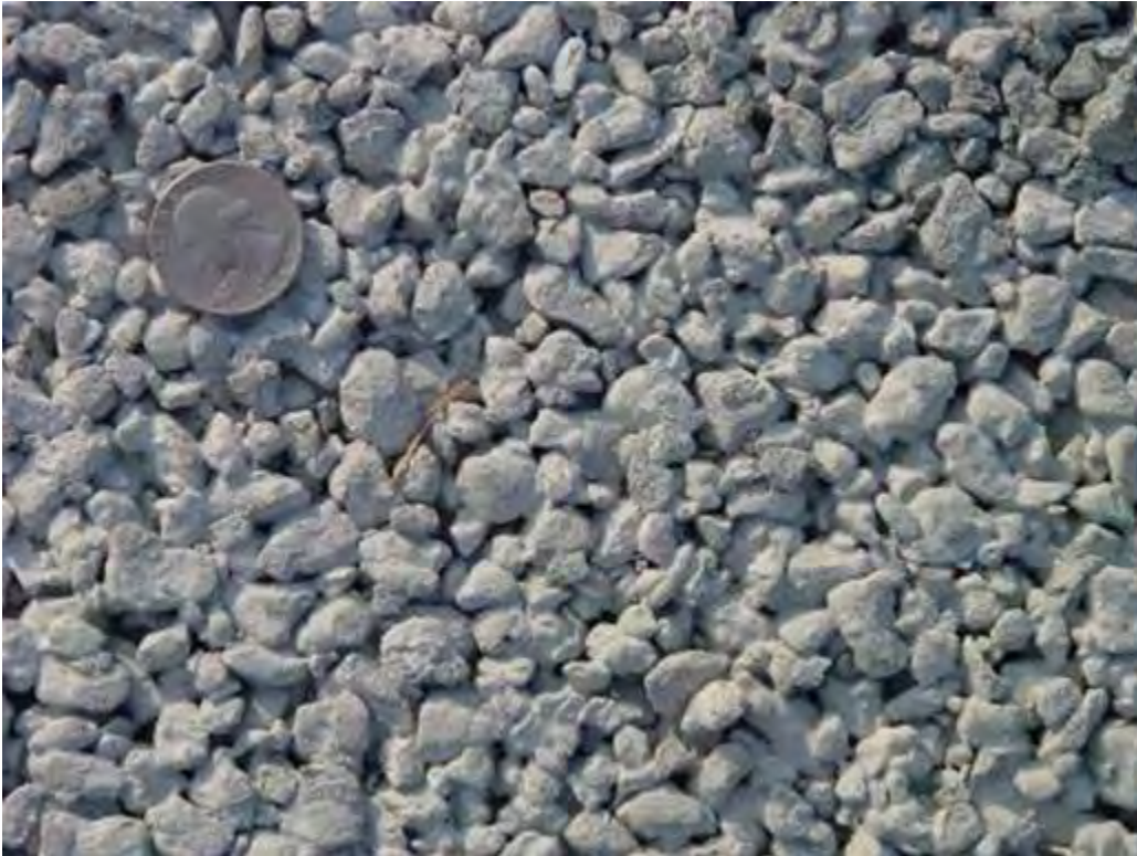
Figure B-3-5. Example of pervious concrete, Kinston, North Carolina. Source: North Carolina State University Department of Biological and Agricultural Engineering
