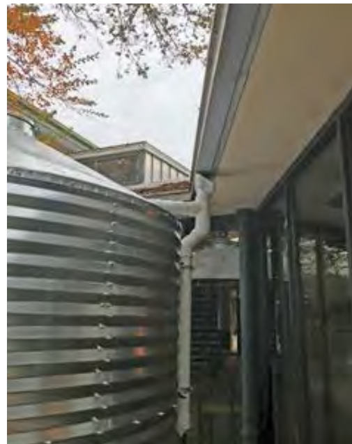
Figure B-9-11. Inlet configuration at the downspout at San Antonio River Authority Main Office, San Antonio, Texas.
