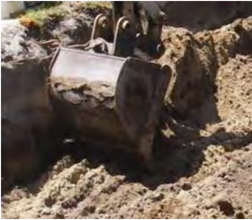
Figure 4-5. Subsoil compaction in an infiltration practice being mitigated by ripping the grade to a depth of 12 inches. Source North Carolina State University Department of Biological and Agricultural Engineering
