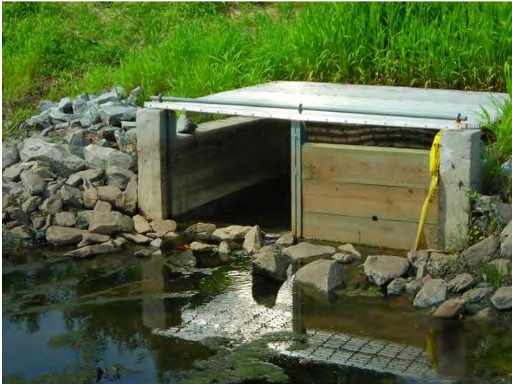
Figure B-7-9. A flashboard riser allows adjustment of water level during plant establishment and for maintenance, Wilmington, North Carolina. Source: Tetra Tech
