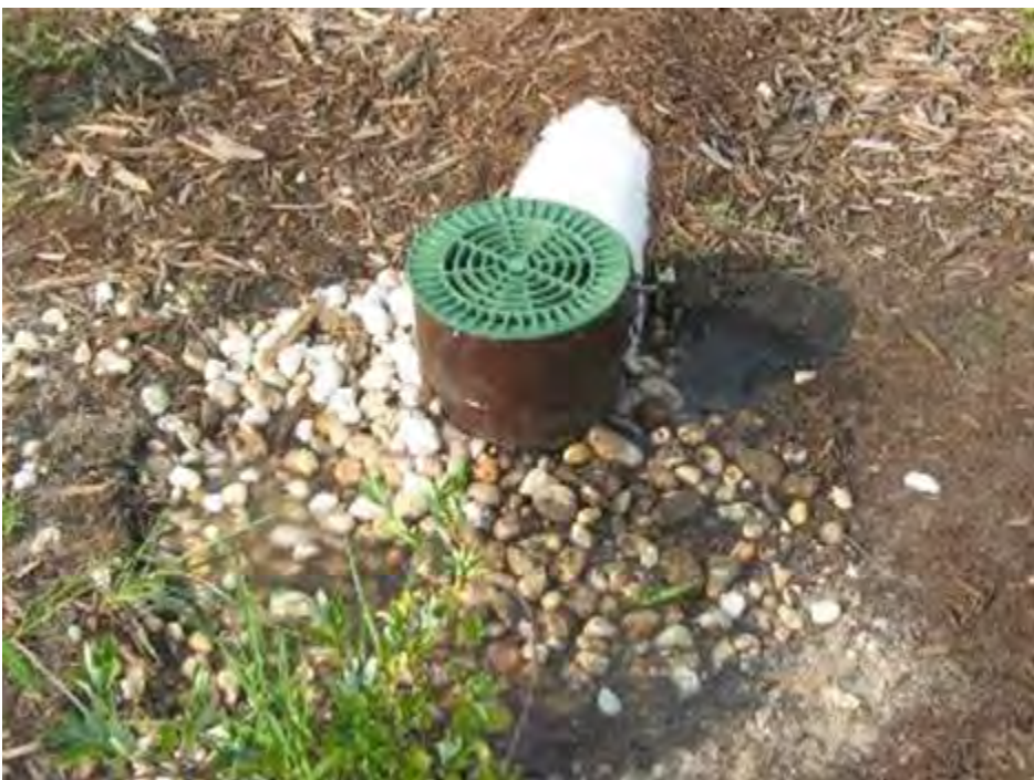
Figure B-1-8. Upturned inlet from rooftop bubbles up diffusely onto gravel pad, Chocowinity, North Carolina. Source: Tetra Tech
