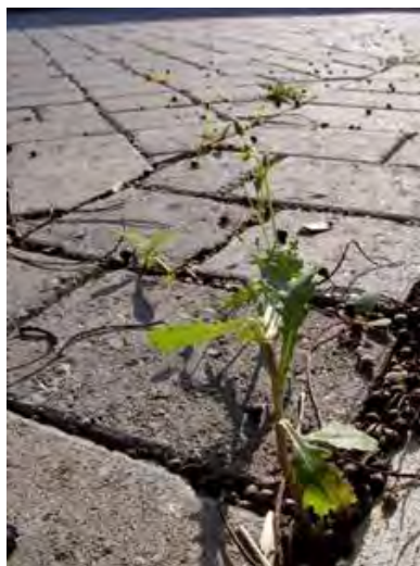
Figure 4-9. Plant growth and debris buildup indicate that permeable pavement is clogging. Source Tetra Tech
