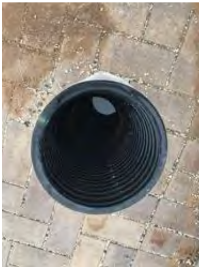
Figure B-3-13. Observation well installed in permeable pavement
