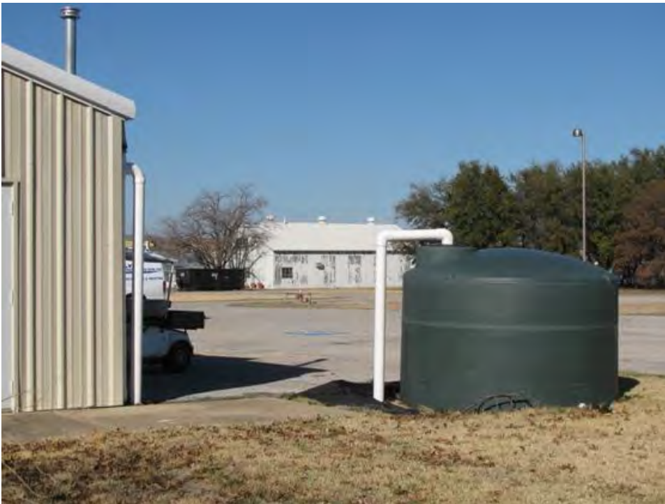
Figure B-9-9. Cistern with a wet conveyance inlet configuration, Dallas, Texas. Source: North Carolina State University Department of Biological and Agricultural Engineering
