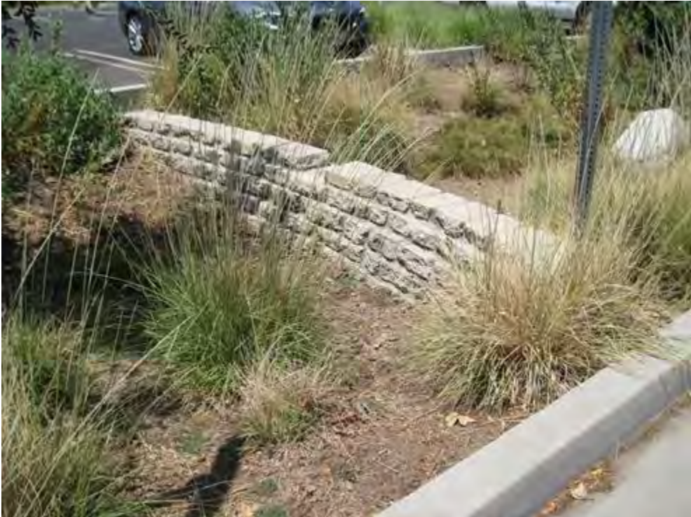
Figure B-2-4. Bioswale with a check dam, Los Angeles, California. Source: Tetra Tech
