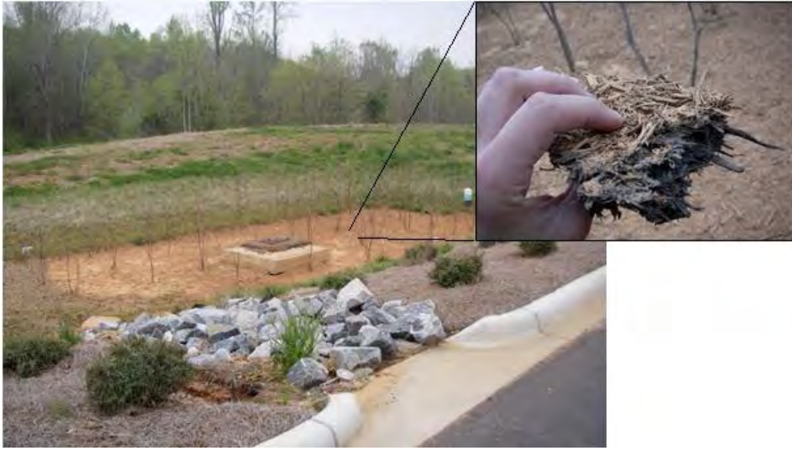
Figure 4-1. Example of a bioretention area installed before permanent site stabilization with the inset photo showing the clay layer clogging the mulch surface. Source: North Carolina State University Department of Biological and Agricultural Engineering
