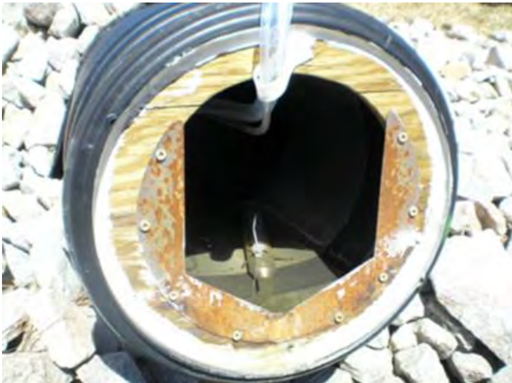
Figure 4-15. Inflow pipe to bioretention area equipped with compound weir and bubbler for flow measurement. Water quality sampling tube and strainer are visible inside pipe. Source: Tetra Tech
