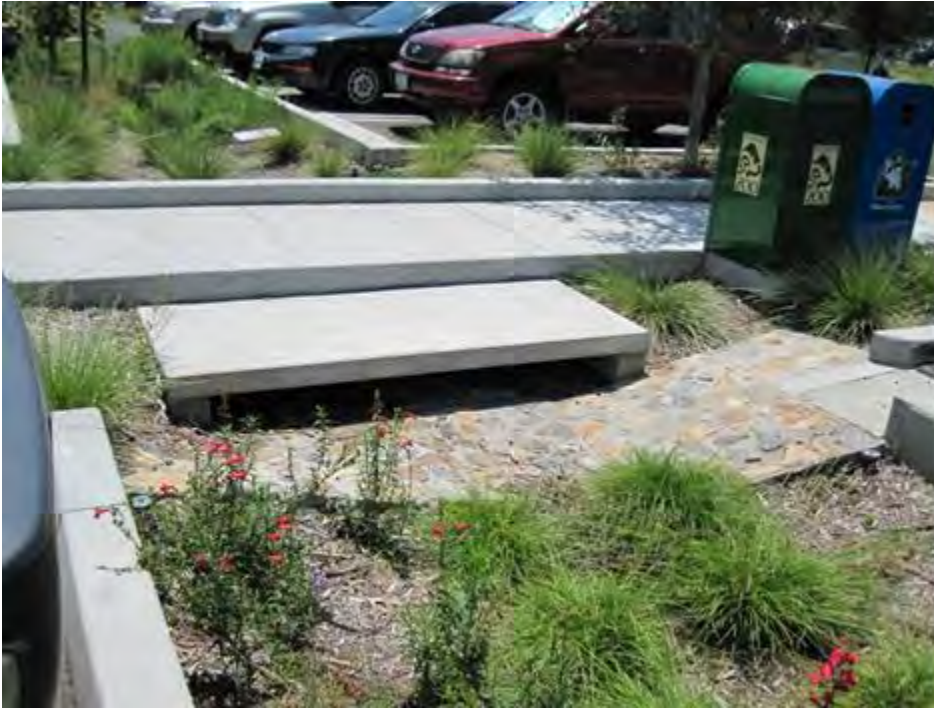
Figure B-1-7. Inlets stabilized with mortared cobble, Los Angeles, California. Source: Tetra Tech
