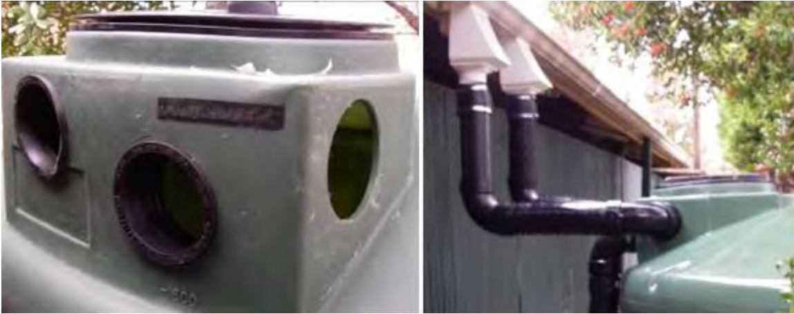
Figure B-9-7. Inlet in the sides of the man way, Greensboro, North Carolina. Source: Tetra Tech
